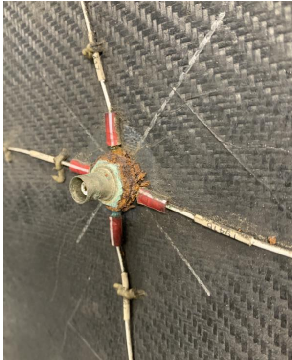
Figure 1 Evidence of Corrosion Underneath the Cowl
