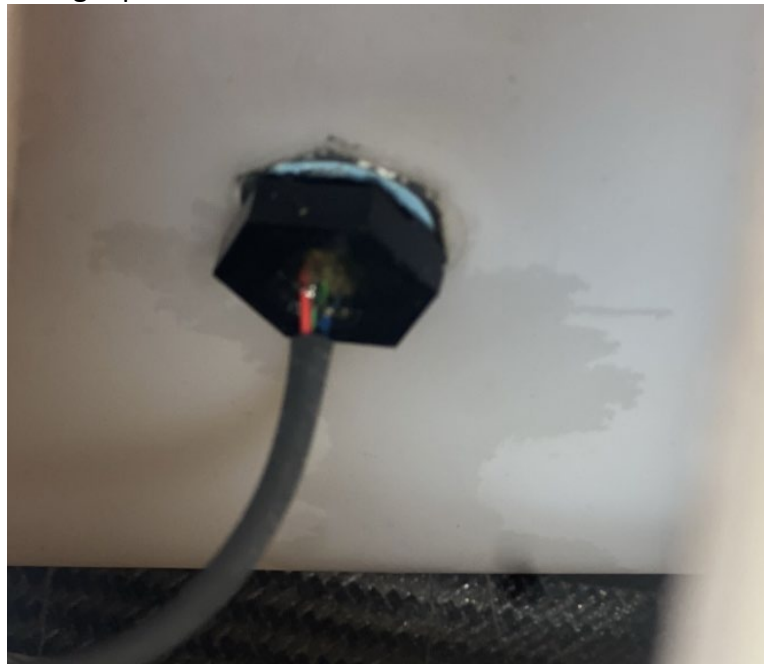
Figure 2. Weeping/Staining around Sensor
